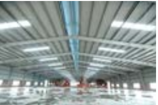
Translucent Panel (Skylight)
